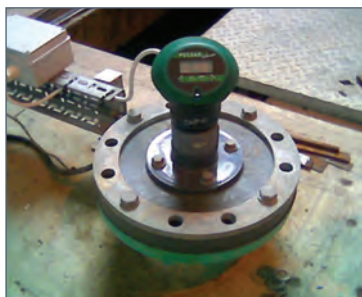
IMP ON A LIQUID LIME TANK
