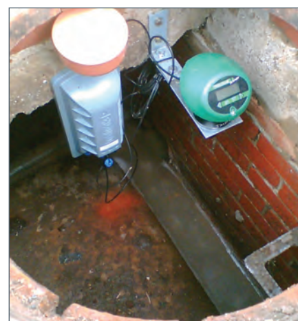
IMP MONITORING IN A CSO CHAMBER
